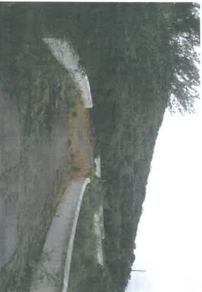
Figure 10: Hodges Bridge in the Cogmans Kloof, built in 1877. This structure is rated as significant and a permit would be required to change or alter the bridge.
