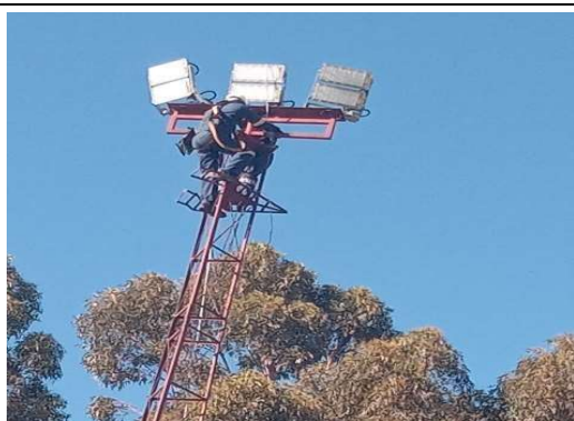
Photo: King Edward sportsground high mast lights.
