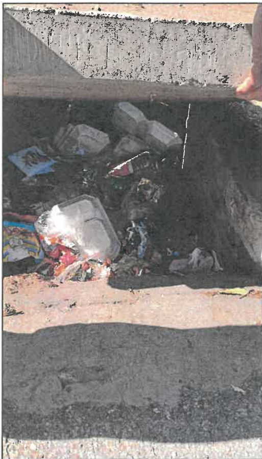
Blocked Culvert in Cross Street
