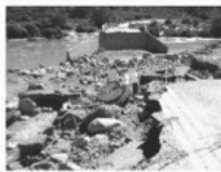
The approach road to the previous Boy Relief Bridge washed away in 2003. The bridge and the pass were rebuilt in 2017-2021 to withstand larger floods.
