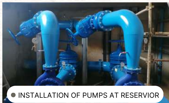
● UPGRADE ROBERTSON WWTW
