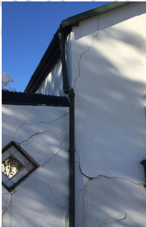
Damage caused by water ingress
