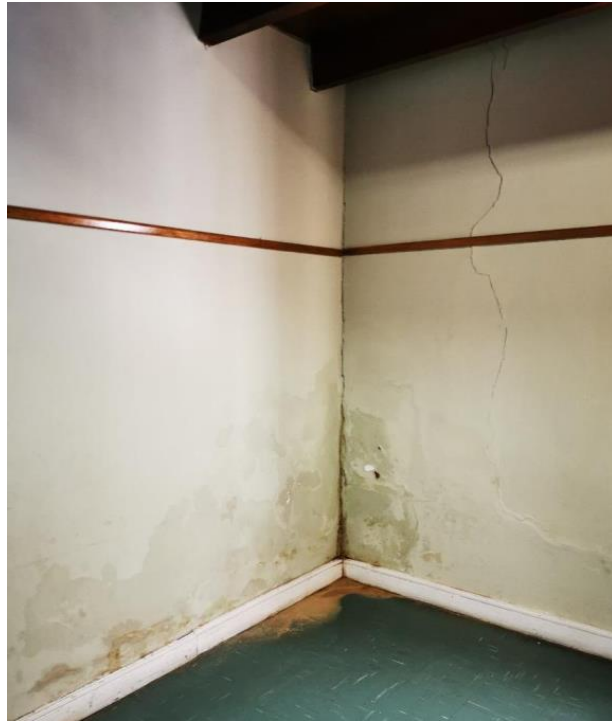
Damage caused by water ingress
