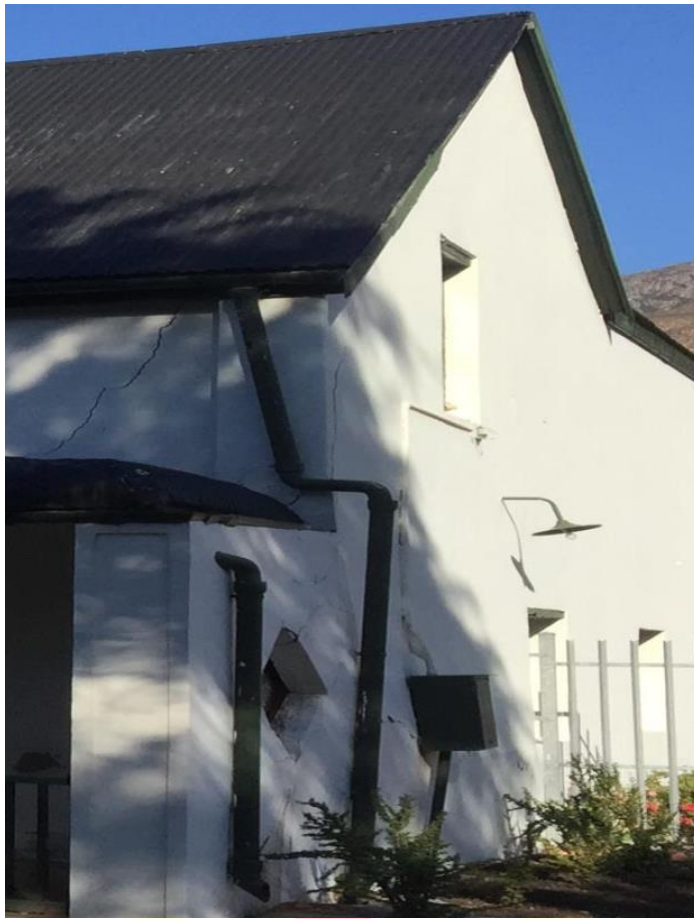
Damage caused by water ingress
